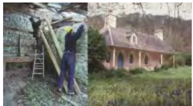
Carpenter and assistant measuring a length of replacement timber in the roof of cattle sheds at Llanerchaeron Farm. The wood will be cut with an adze beforehand and pegged with wooden pegs. The charming C18th Estate Office at Llanerchaeron, set in a field of bluebells. The rough stonework of the cottage is painted pink and white and the windows and doorframe are arched.
