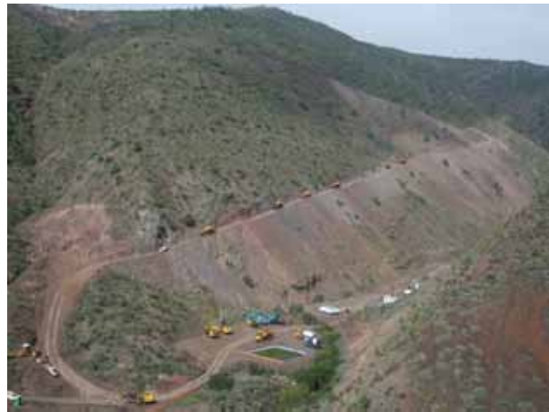
St Helena Airport haul road: Rupert's Hill to pipe ridge – climbs 300m over 5km
