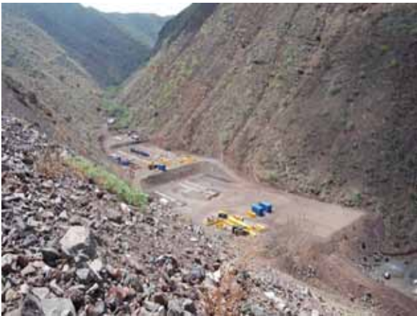
St Helena Airport bulk fuel installation
