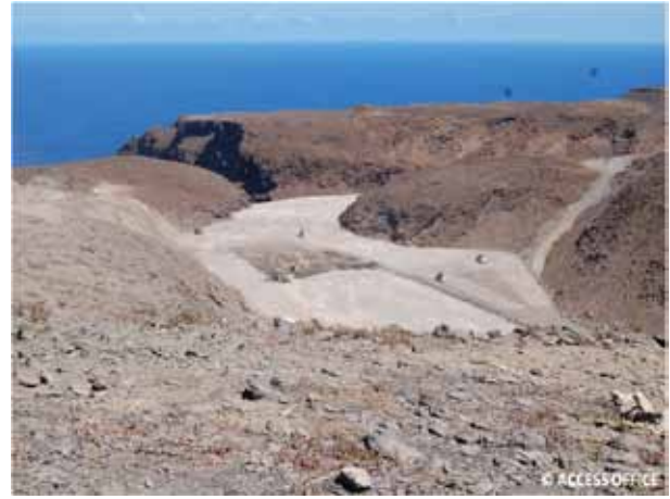
St Helena Airport Dry Gut infilling: 7.6 million cubic metres of rock dumped and compacted to maximum height of 120m
