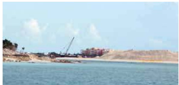
Coastal destruction, including mangroves, during the hotel development at Leeward.
