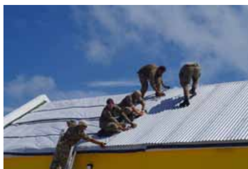
Right: Royal Marines repairing the roof of the Salt Cay airport building.
