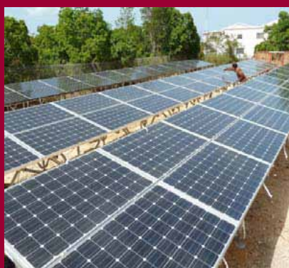
Solar installations at the Hughes Medical Centre: top - roof-mounted, bottom - ground mounted. Photo: ARIEP
