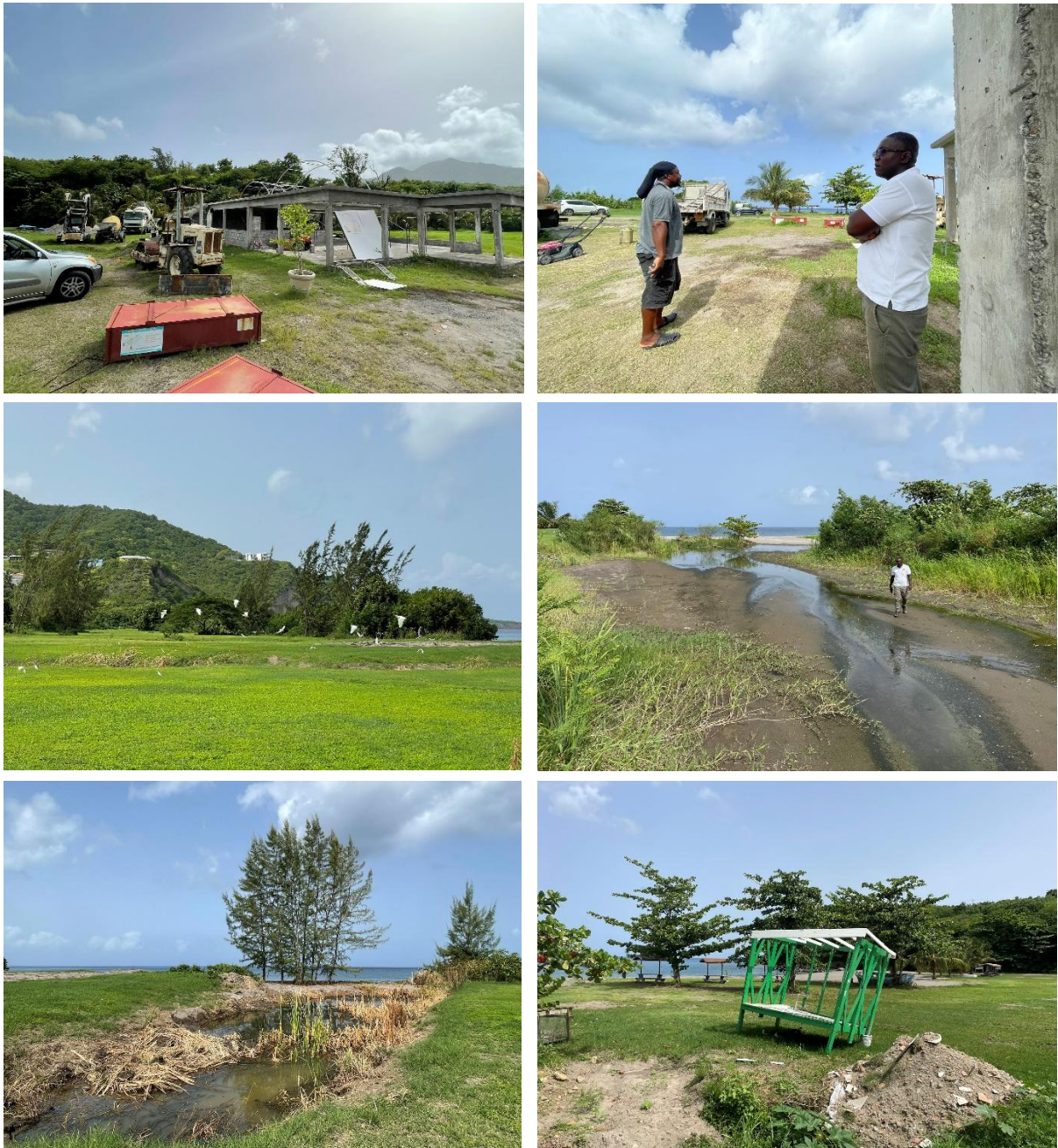
Figure 12 - Top left: The framework of the beach bar under construction. Top right: Chris and Dwayne on the beach bar construction site. Mid left: Little Egrets in flight over the lowland area that changes in topography regularly with storms and water flow across the site. Mid right: Chris on the existing river channel approaching the sea in the background. Bottom left: The remaining small pond on the site (much reduced in size following a recent storm). Bottom right: The remains of the bird viewing platform built by Dwayne and funded by the RSPB.
